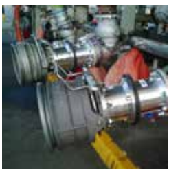
Oil and gas flow control
